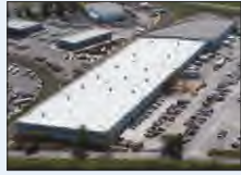
Hunter Douglas Fabrication, Sacramento (CA), USA
