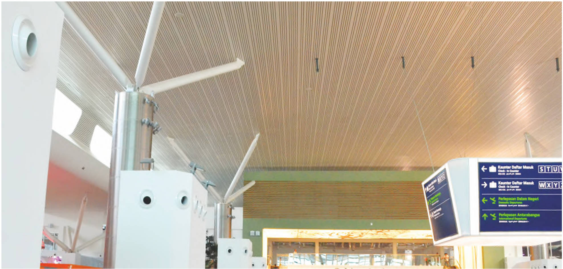
KLIA2 Malaysia Multi B ceiling
