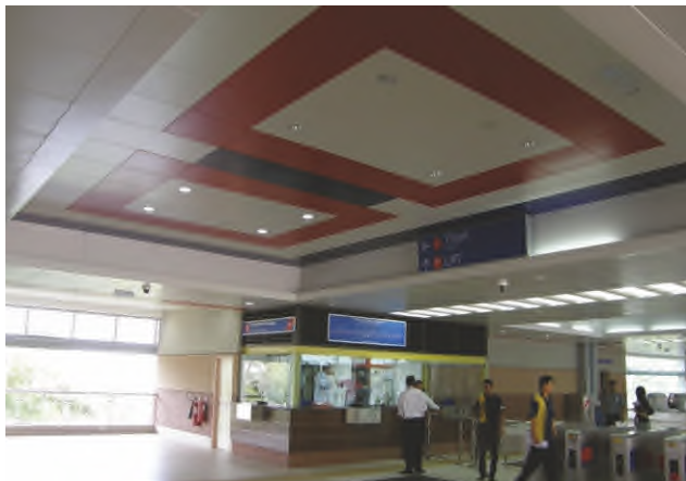
LRT station@Sri Rampai, Kuala Lumpur, Malaysia Clip-in Tile ceiling
