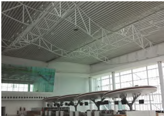
Sepinggan Airport Balikpapan, Indonesia 150C Ceiling
