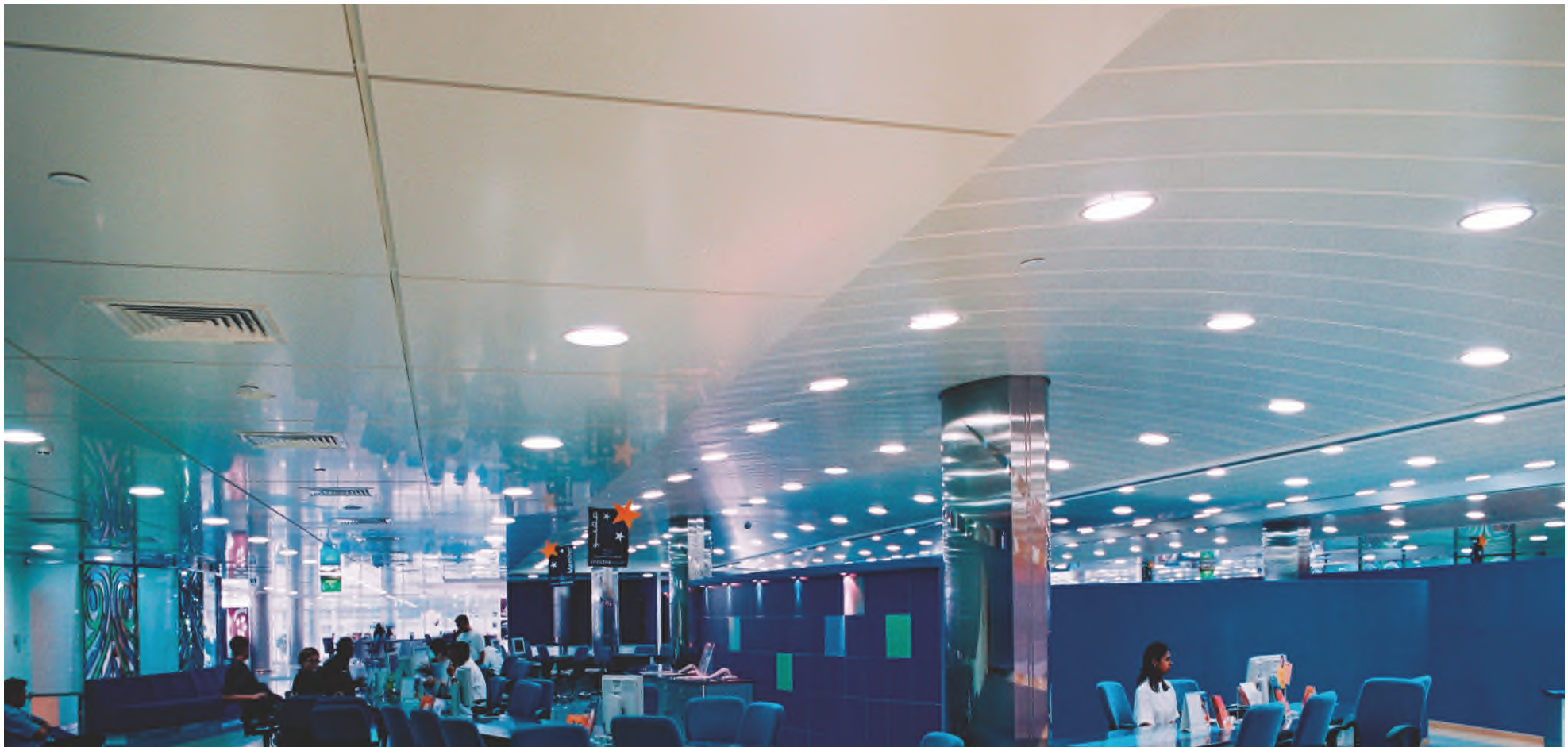
Dnata Airline, Dubai Lay In Tile Ceiling
