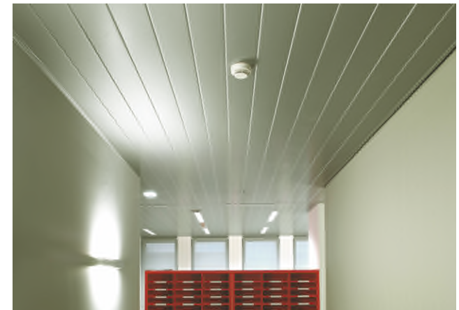
InBev Brewery, Belgium 150C ceiling
