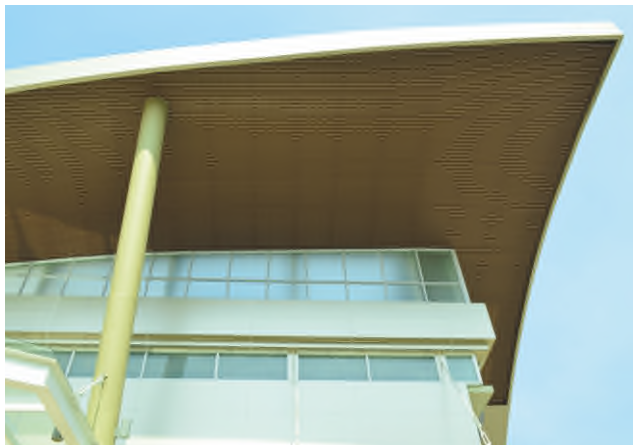
Sasana Kriya Convention Hall, Jakarta Indonesia 84R ceiling
